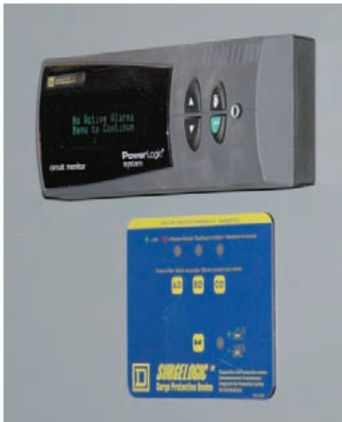
Power monitoring and protection devices.
