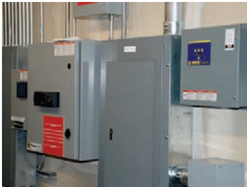
Permanently installed monitoring and protection system
