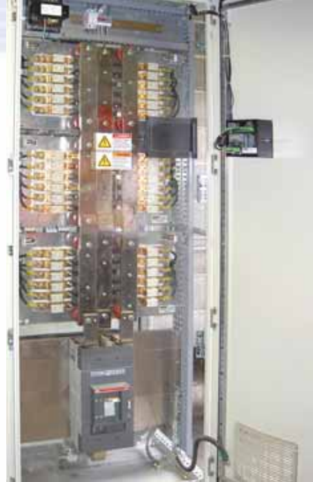
Internal view of enclosure, 600 kVAR with molded-case circuit breaker.
